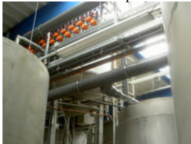
Pipework and distribution systems
