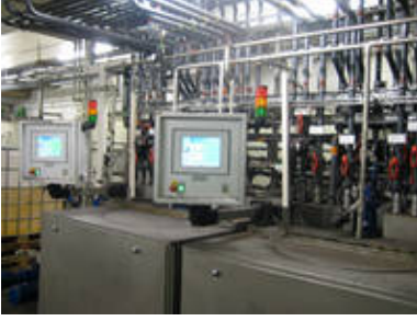
Chemical dosing systems
