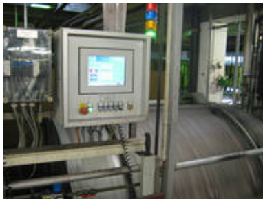
Drum - control systems
